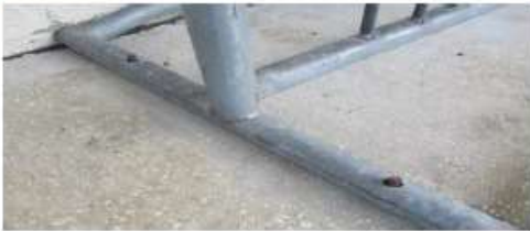
2 – Fixture needs to be re-anchored
