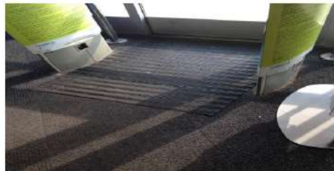
Soft grid missing fasten (grade = 1)
