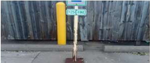
1 – Replace posts due to damage or excessive rust
