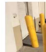
Bollard Cover damaged; Bollard leaning, assume grade = 1
