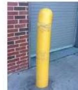
Bollard Cover damaged; Bollard upright, assume grade = 4
